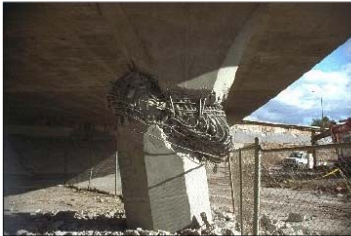
Figure D-15 Earthquake Damage (Source: FEMA)
